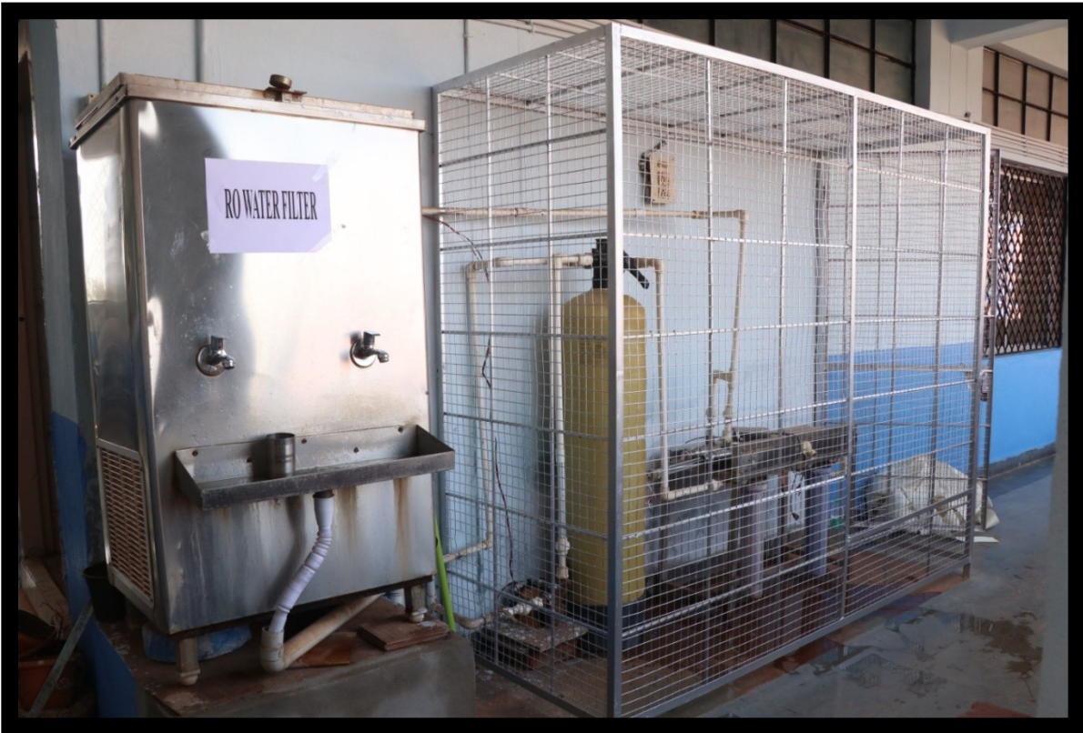
RO Water Filter (UG)
